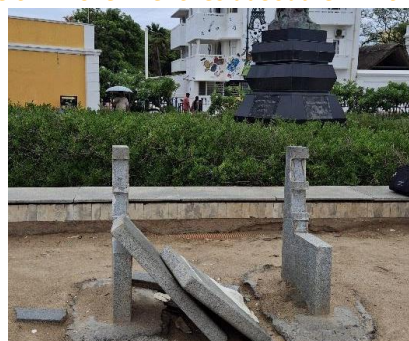
Figure 62: Broken Benches at Southern Promenade
