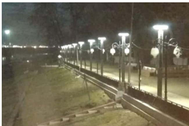
Figure 15: Lighting installed along riverbanks
