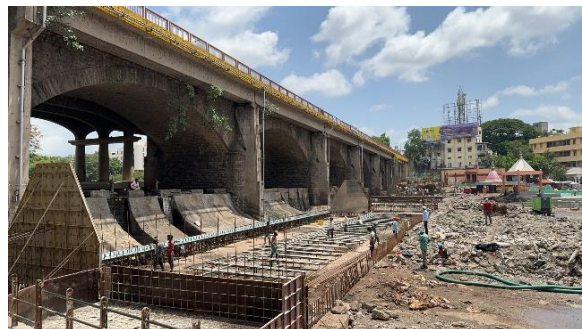
Figure 47: Construction of foundation for Pneumatically operated automated mechanical gates at Ahilya Bai Holkar bridge
