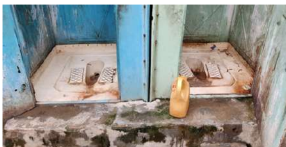
The state of the pre-fabricated toilets (provided by the govt.) in the settlement.
