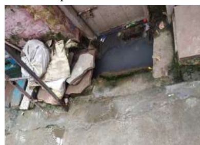
Wastewater entered in the house due to overflowing drain
