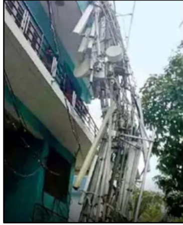
Image 8 Collapsed telecom tower erected on top of a two-storey building, Thoppumpady Source: timesofindia.com
